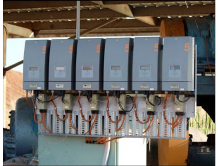
A bank of six inverters change solar-generated power from DC to AC so it can be used by the adjacent pump or fed into the grid. Solar power on this site is supplied by a 30kW array of panels.
