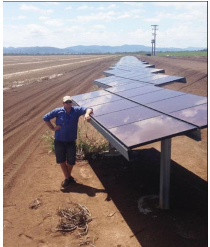
Scott Morgan with his 160-panel solar array which generates 9.6kW of power. On sunny summer days, it is capable of producing 70kW hours per day of energy, and averages 40kW per day for the year.
