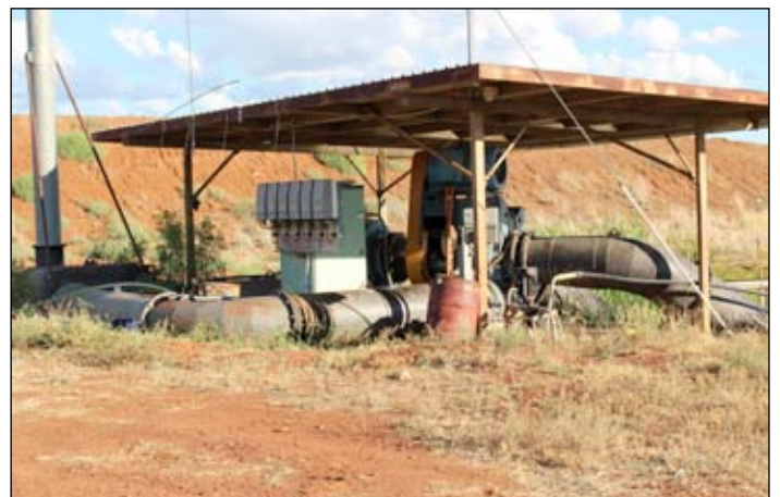
Pump located at St George grower Ian Brimblecombe's property. Photo courtesy: Seedbed Media.
